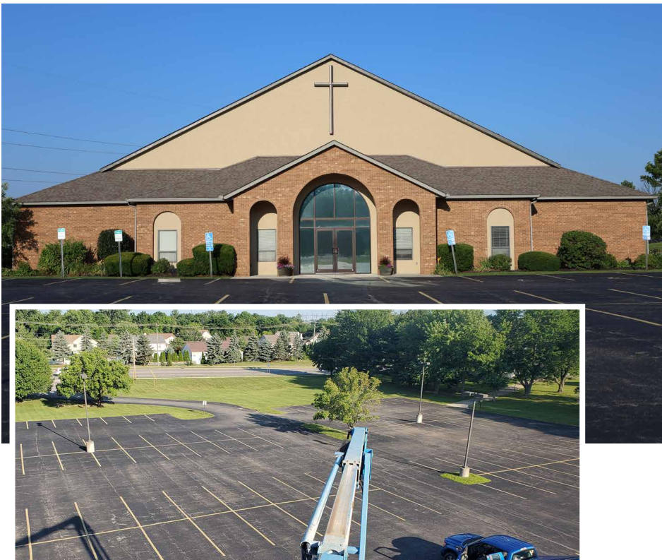
At top, the finished job with the evening sun reflecting off the cross, and a brighter and cleaner look to the church exterior. Bottom, a view of the parking lot that not many have seen, except perhaps for our feathered friends who build their nests each year in the nooks and crannies in the ceiling of our front porch. Thanks to Dan Brill for the selfie on the front and the bird's eye view above, and to Rachel Cherubini for the photo on the front of Dan at work.
